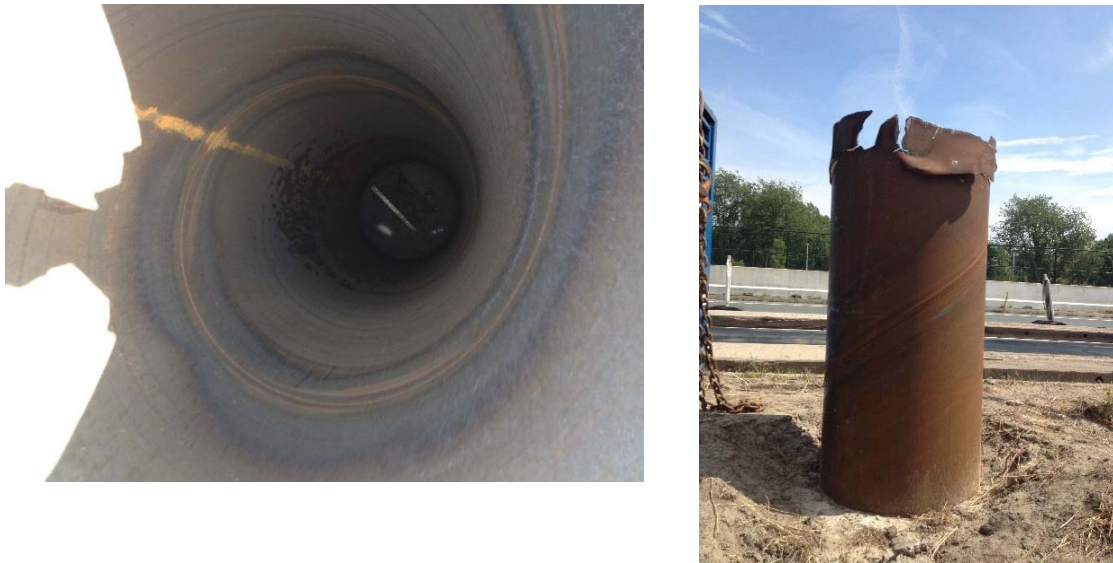
Fig. 8: soil plugging within a pile and pile top damage due to extensive vibro driving
